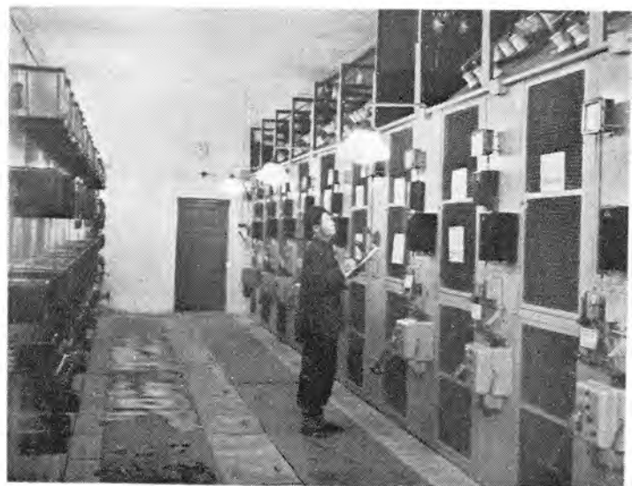
Switchboards in the central control room
